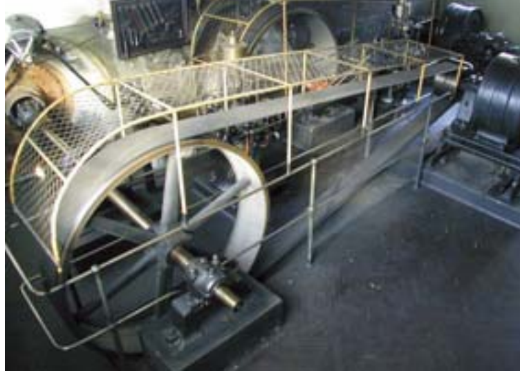
The old Titan hydroelectric power station was built in 1920, and it is still in a perfect working condition producing enough electricity to cover a great deal of the needs of the new Titan factory.
